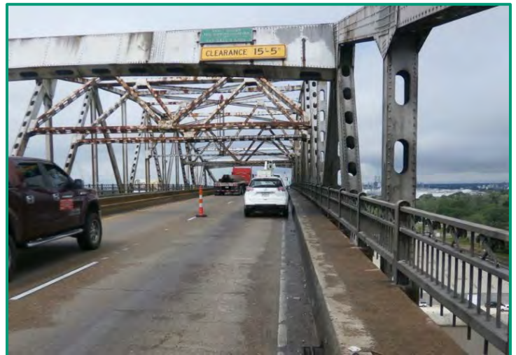
Figure 8: No Shoulders and Low Vertical Clearance
