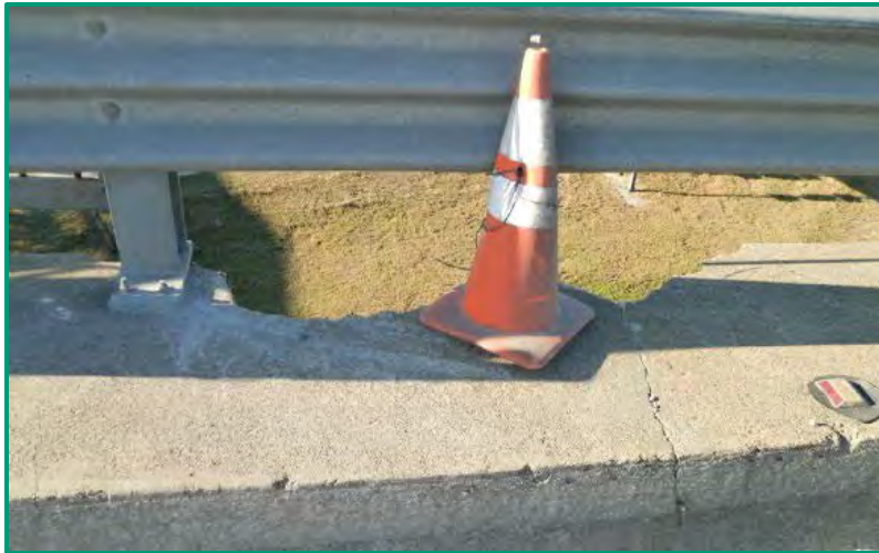
Figure 5: Large Spall in Bridge Overhang
