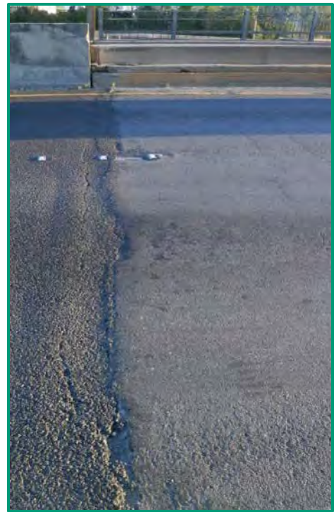
Figure 6: Typical Widespread Traverse Cracking in Bridge Deck
